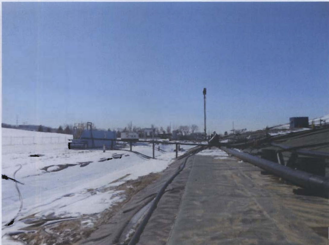
14. Flare station and frac tank located on SE side of landfill.
