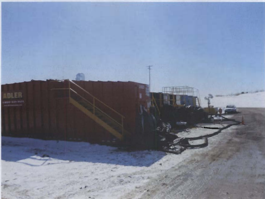
24. "Approved" frac tank storage for treated leachate.
