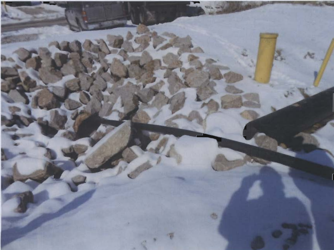
34. Area of 2-9-14 leachate release; inlet of storm water culvert that drains to Outfall 003.
