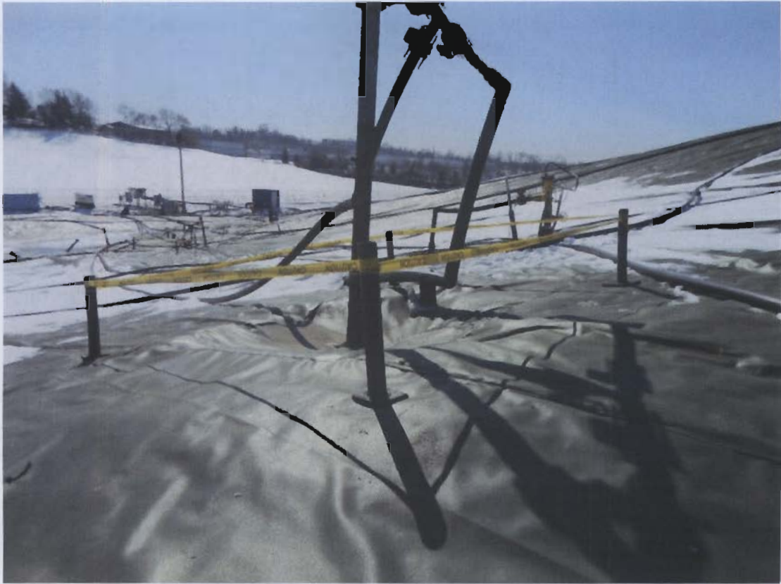
1. Subsided are #1 located at GEW-64A.
