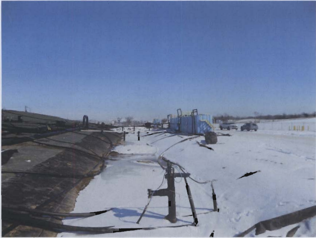
15. Frac tanks located on SE side of landfill.
