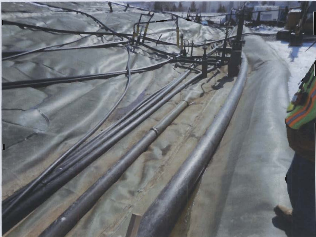
32. Area of 2-9-14 leachate release at SW corner of landfill; leachate accumulated under liner.
