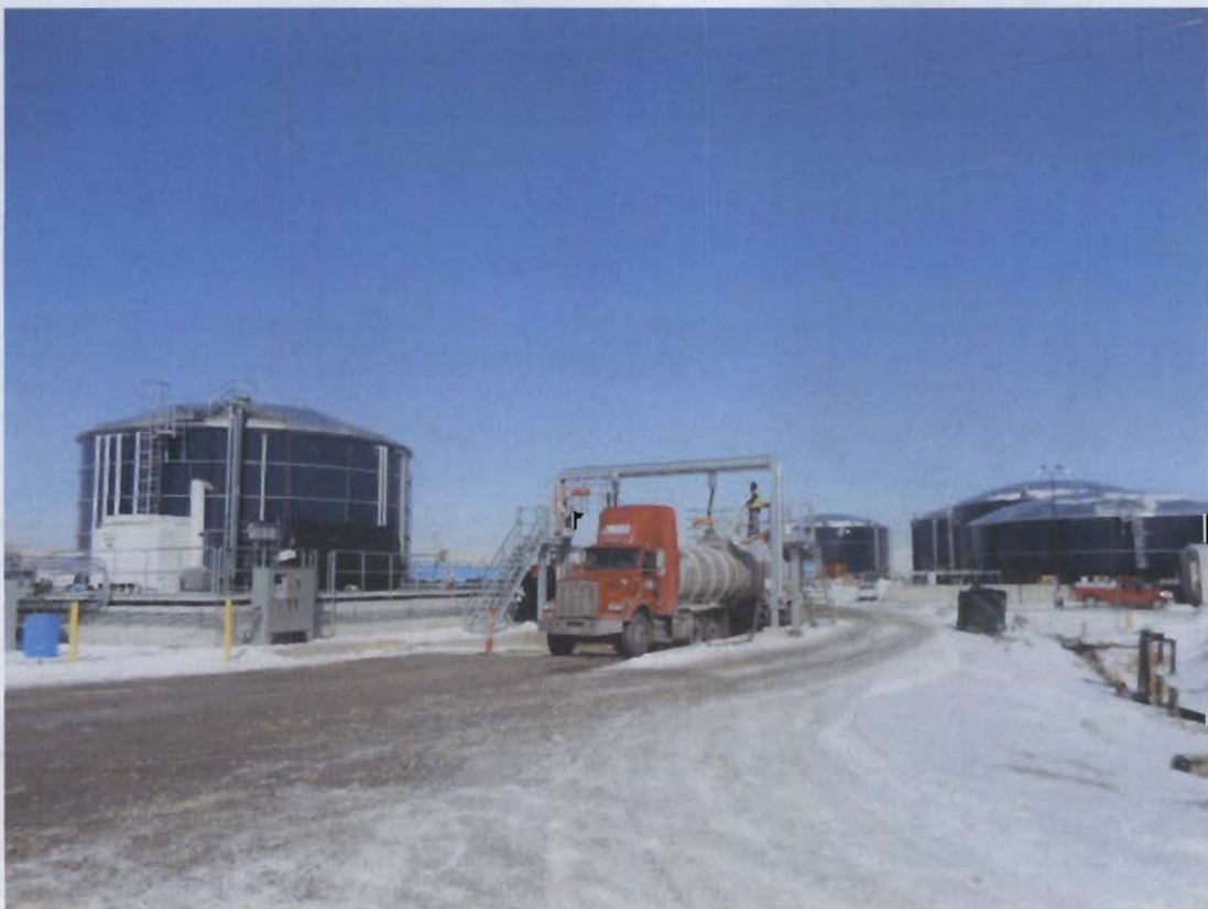
20. 316K leachate treatment tank and truck load-out station.
