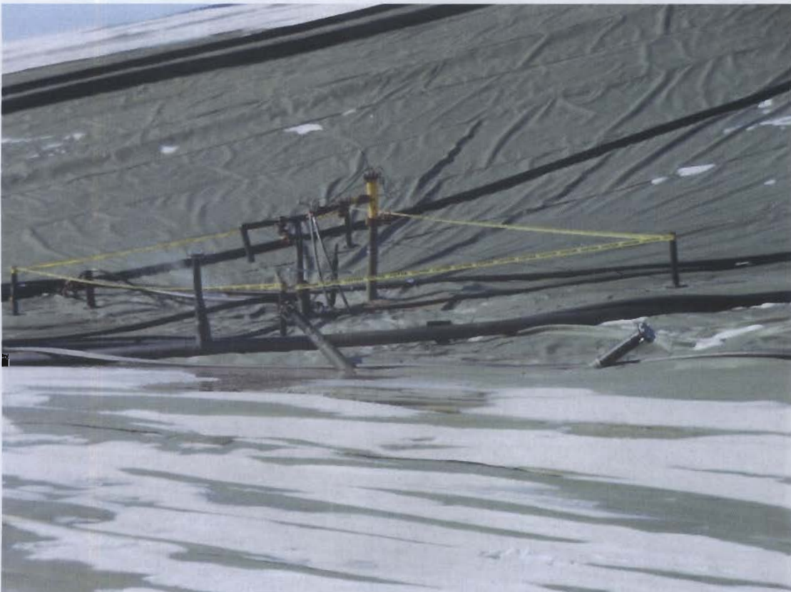
2. Subsided area #2 located at SEW-31R.
