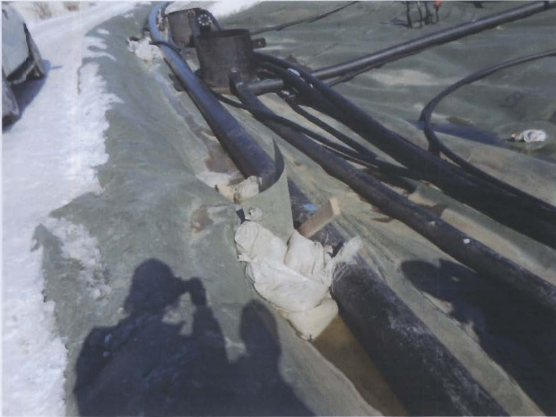
33. Area of 2-9-14 leachate release; inlet to storm water culvert (currently blocked).
