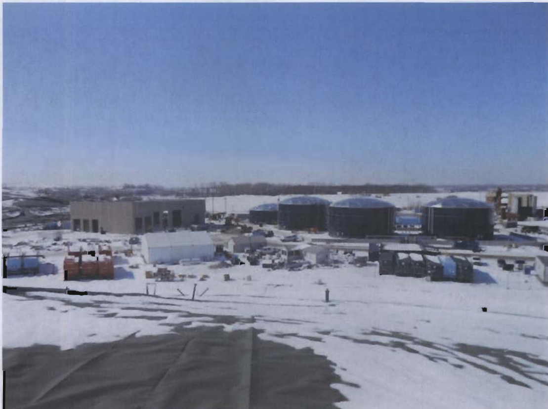
18. Emergency storage frac tanks (16) and vac-truck storage building; leachate pre-treatment plant and I-M tanks in background.
