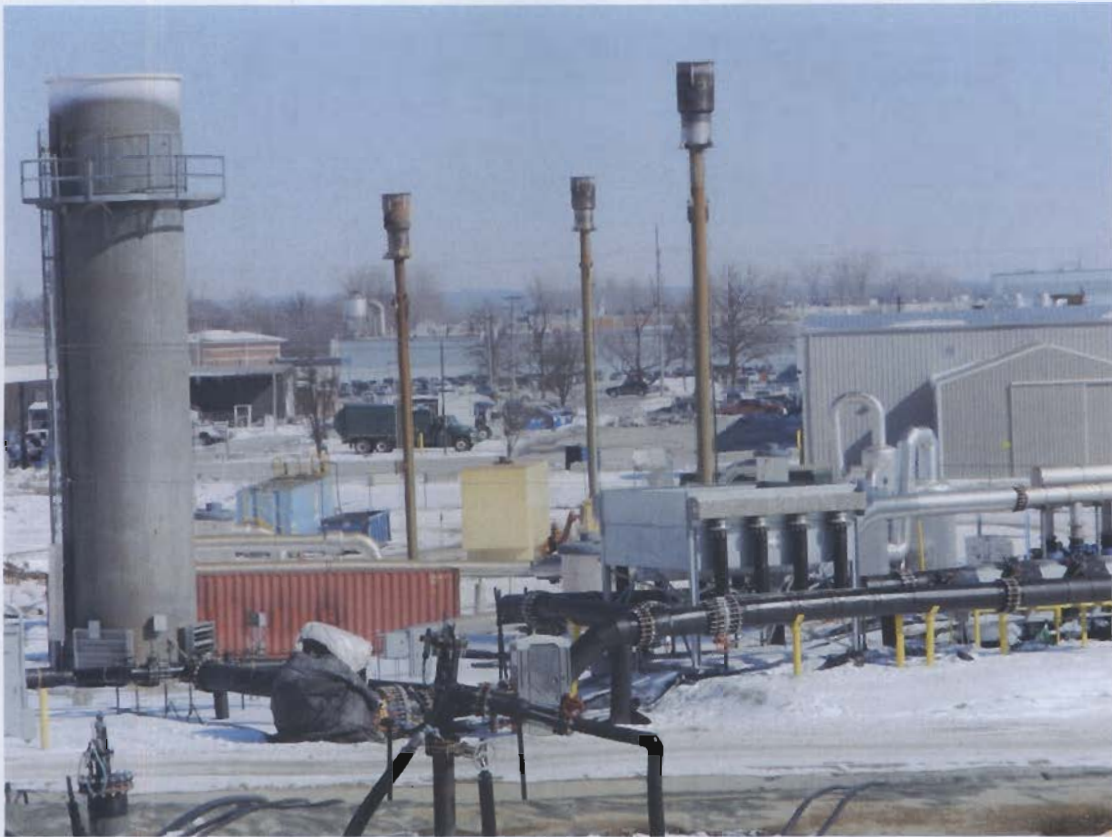
25. Three candle-stick flares at main flare station; former enclosed flare on left.
