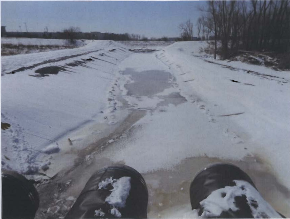
31. Recently lined swale between road and SW sedimentation basin; leachate from spill still present.
