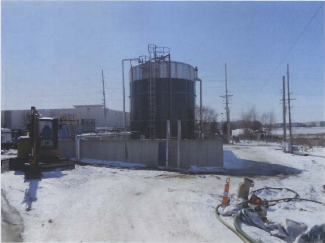
23. 96K tank at SW corner of landfill; MSD lift station in background.
