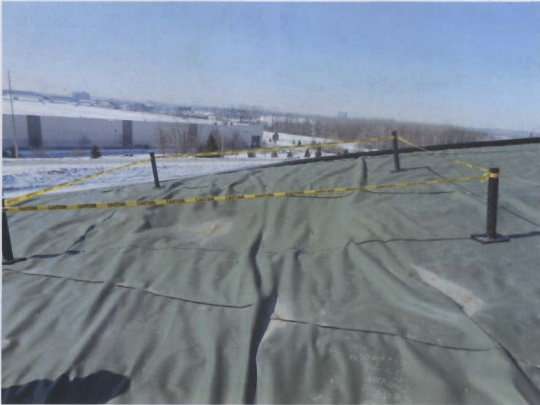
3. Subsided area #3 located at former LCS-2 (near GEW-26R).
