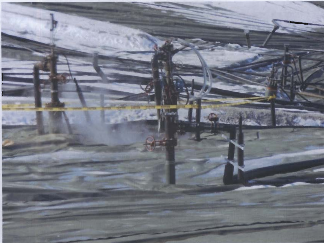
6. Subsided area #6 located at SC-1.
