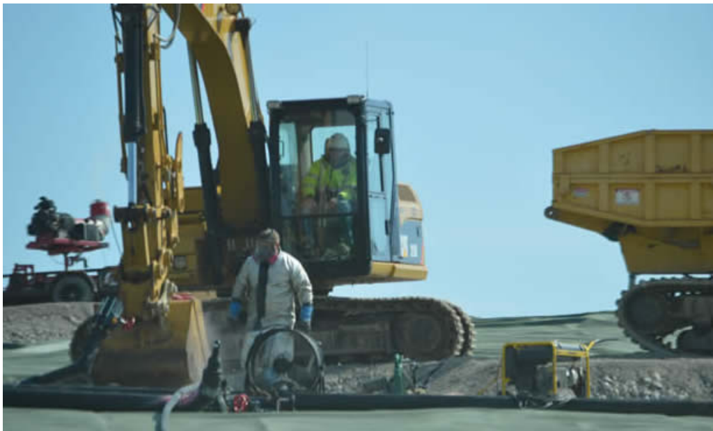
Photo of work on gas extraction well (GEW-21) on the south slope of Bridgeton Landfill, May 16, 2014
