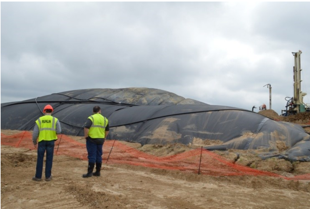
Photo 4. Excessive Landfill Gas and Inflated FML, May 2013 (Source: DNR Staff, 2013).
